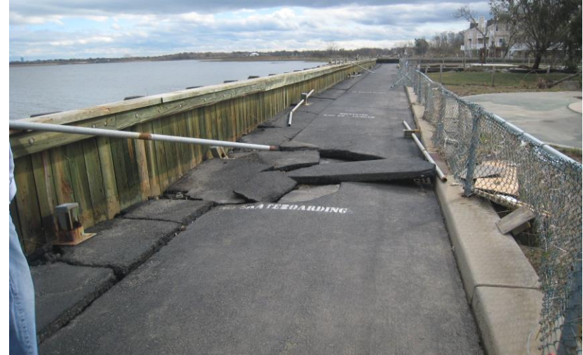
Figure 14: Damage to the Walkway along Firefighter's Park
